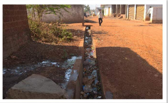
Picture 5: Clogged drain in Naubad area
